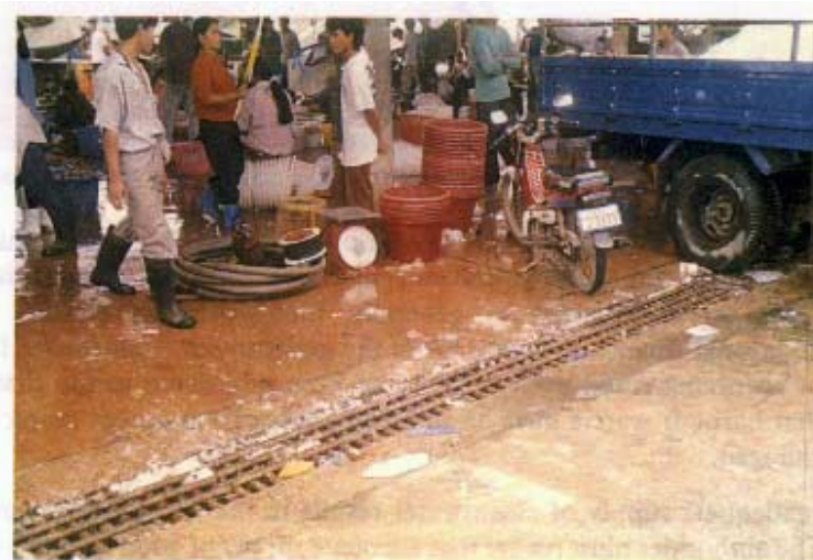
Drain for waste water from landing/cleaning pier at the FMO Port, Phuket
